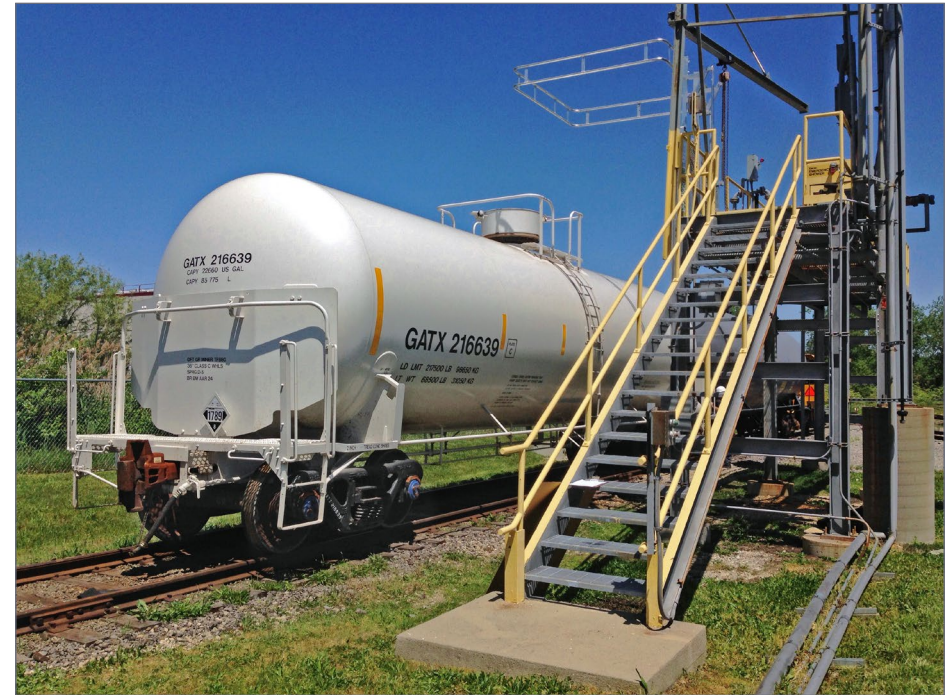
2. An excellent example of simple unloading rack in a small transloading facility. Chlorine Institute photo
