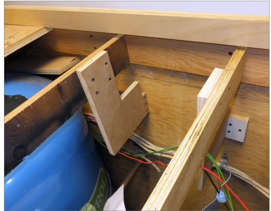
8. The pesky blue water pressure tank that has plagued many of my layout efforts was at it again! There was only one way to get two tracks to pass underneath Tunkhannock, and that was to sneak them behind the tank near the top. Clearances were tight – I just made it. The strange L-shaped plywood brackets were created so that I could chop off the existing joist ends. This was the area the new tracks needed to pass through.
