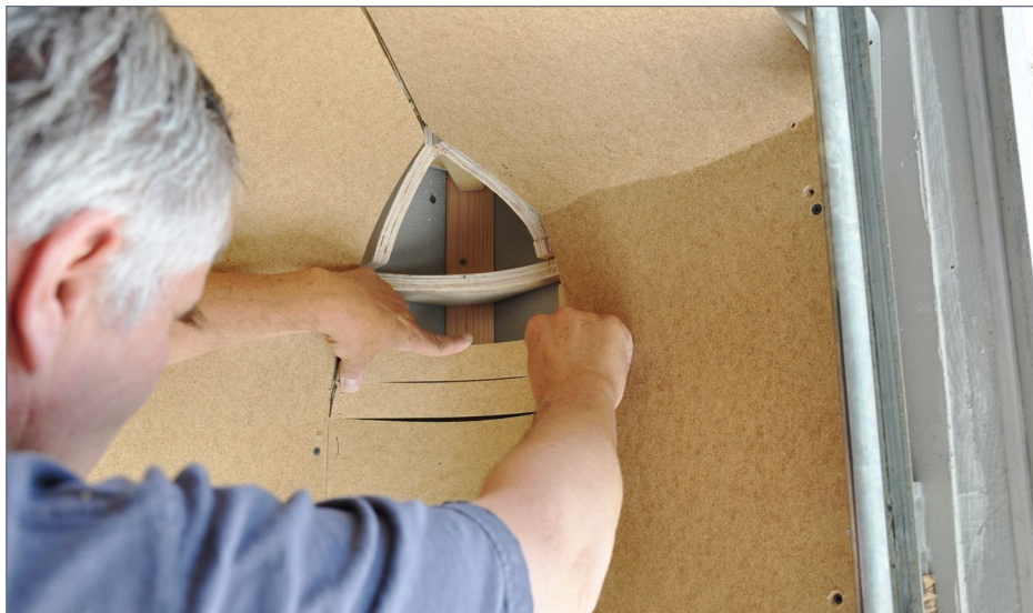
11. I filled in the corners with small pieces of Masonite, test-fitting each piece before I nailed it in place.
