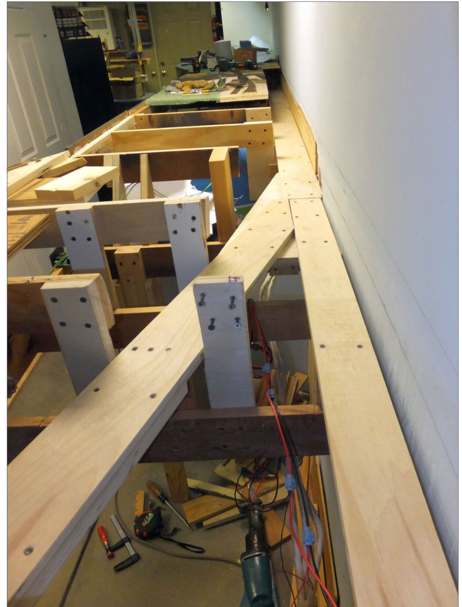
12. Ready for track! The new pathway to the lowered staging yard is in place below Ransom and Tunkhannock.
