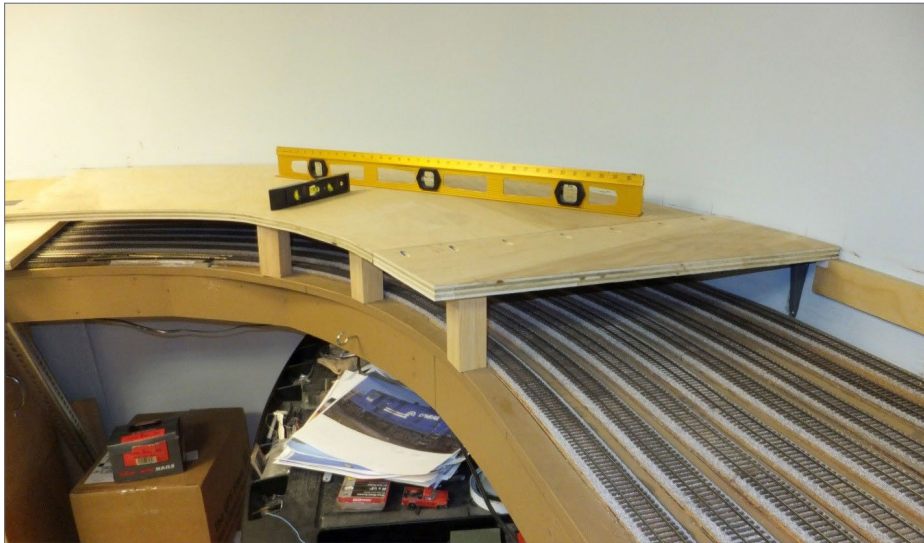
19. Wooden blocks are used as temporary supports for front of the new segment. You can't have too many levels for this kind of work.
