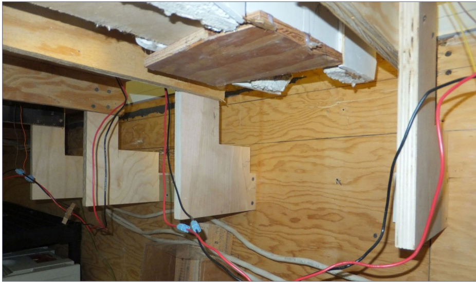
11. Viewed from underneath, you can see the "slot" created where the new pair of tracks will be installed in the cut-out of the L bracket.
