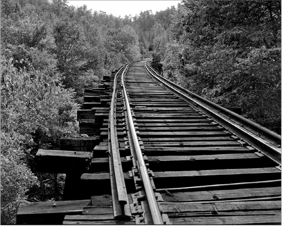
27. Twin Seam Mining Company - 5th Daniel Creek Trestle. View west from end of tunnel 3 across the fifth trestle up Daniel Creek. East end of tunnel 2 is in the distance. This trestle is about 350 feet in length. Note guard rails are on the outside of the running rails. William G. Gordon photo
