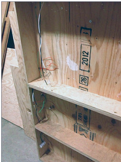
4. I completed the wiring and turnout controls while Pembroke II was still in the garage and could be easily stood up on its end or side.
