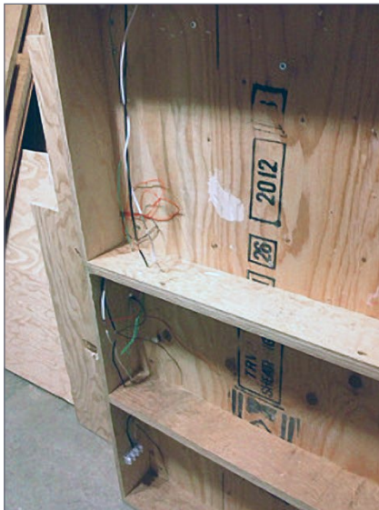
4. I completed the wiring and turnout controls while Pembroke II was still in the garage and could be easily stood up on its end or side.
