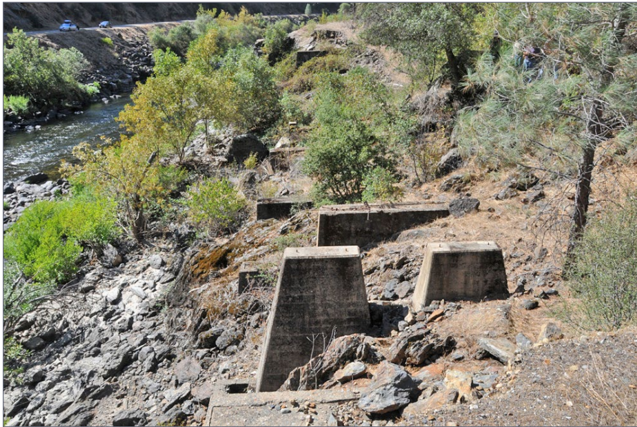
7. The second set of piers from the abutment at the bottom of this photo shows a very short pier for the trestle post nearest the river while the rest of the pier is taller for the other three posts.
