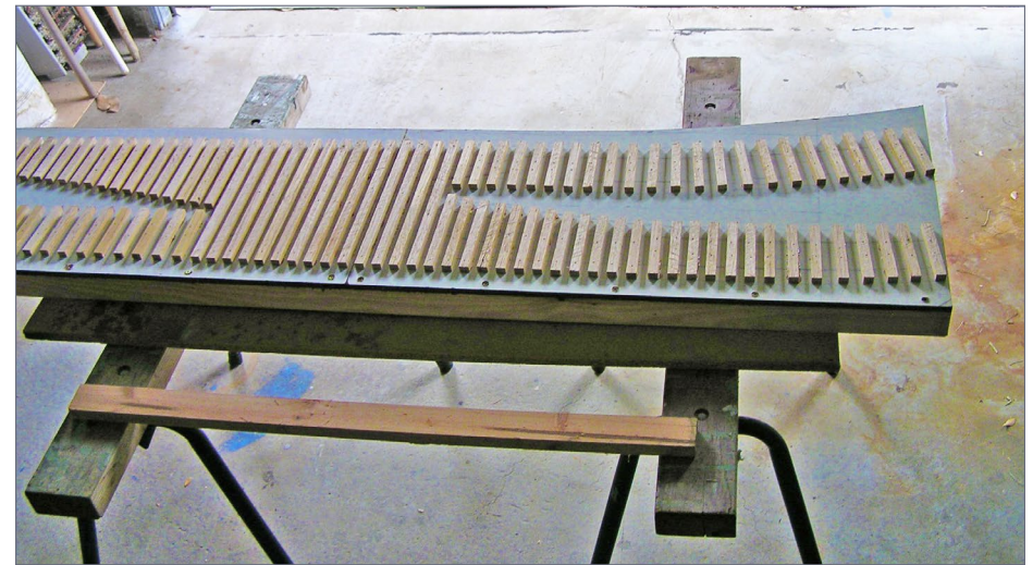
2. I set the turnout on a pair of work benches for ease and comfort spiking the rails to the ties.
