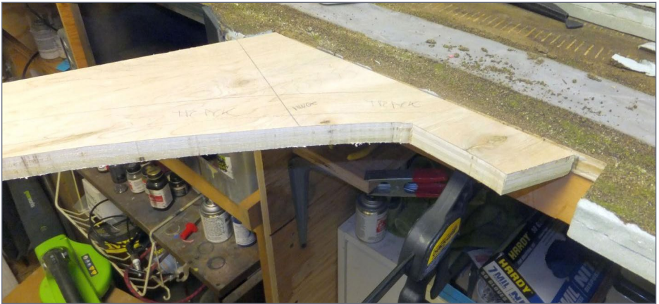
28. The new sub-roadbed is now continuous from staging across the aisle onto the layout in the distance. Note that the bridge hinge and latch points have not been cut at this time.
