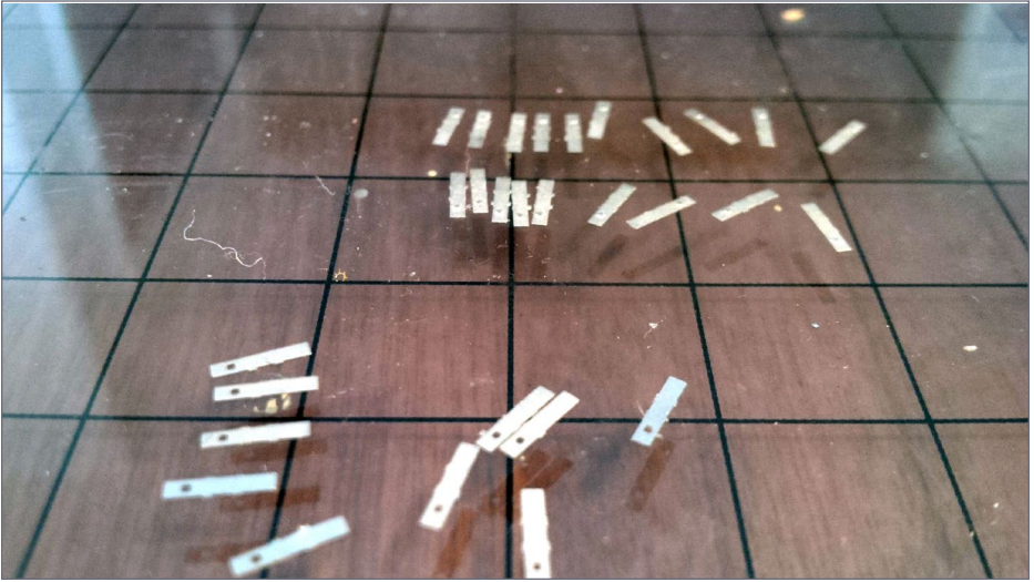
29. The frog tie plates have been cut out and readied for installing.
