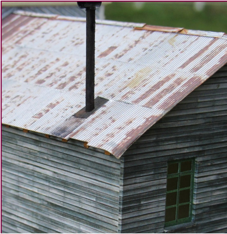
6. Distressed roof and ridge covering.
