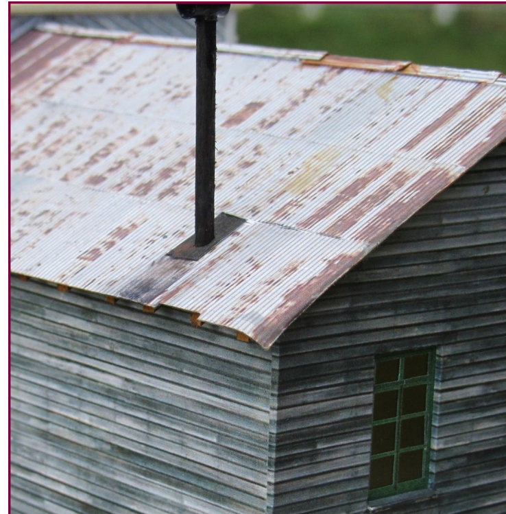
6. Distressed roof and ridge covering.
