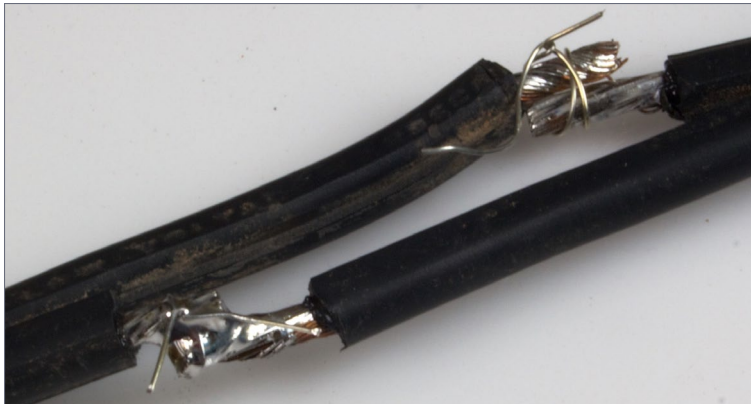
14. Butt splice in bus wire. Lower left has been wrapped with smaller solid wire and soldered. The
