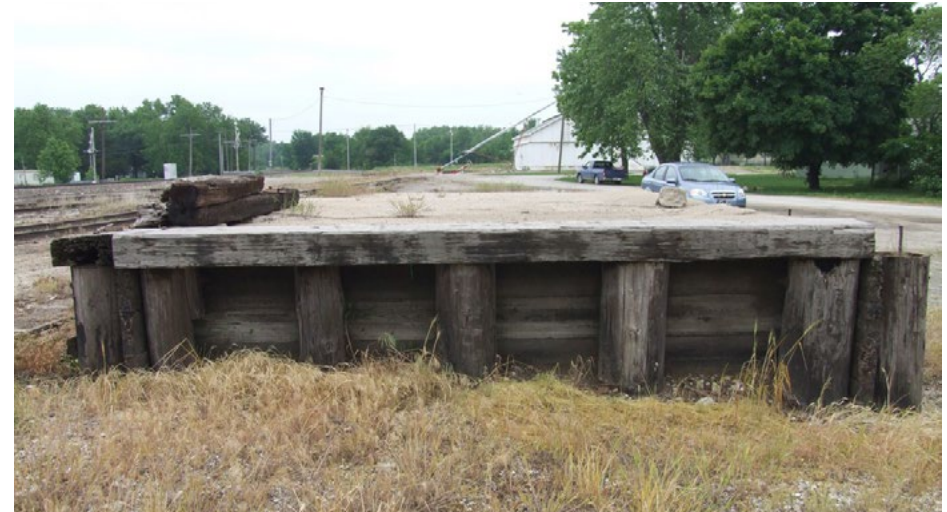
5. The platform end of the dock, looking south. Note the heavy timbers used as a top chord, and also where they are missing on the dock's sides. Also notice the heavy round poles used to support the structure. May, 2008. Photo by Jared Harper
