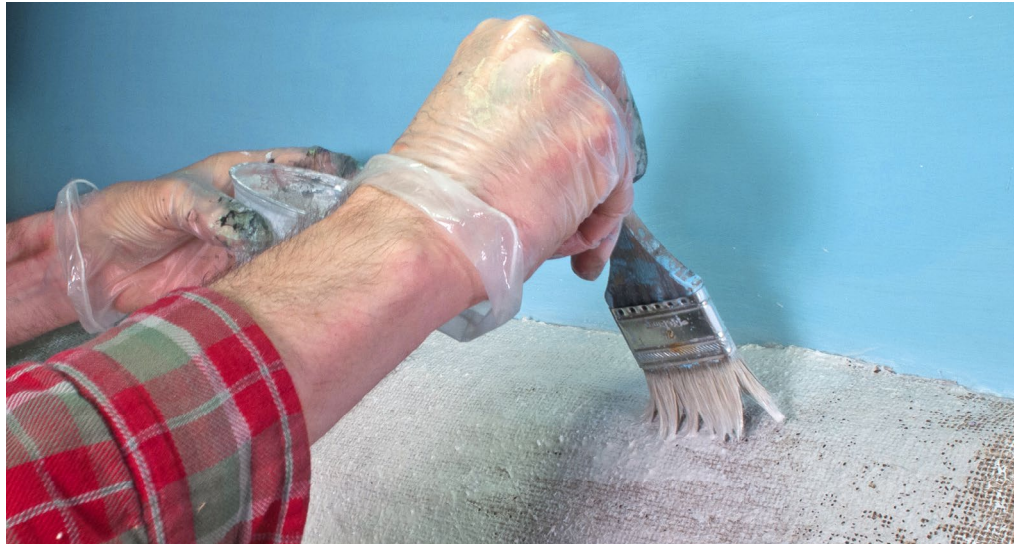
12. The dried plaster contrasts with the second darker layer, allowing you to see where coverage is needed.
