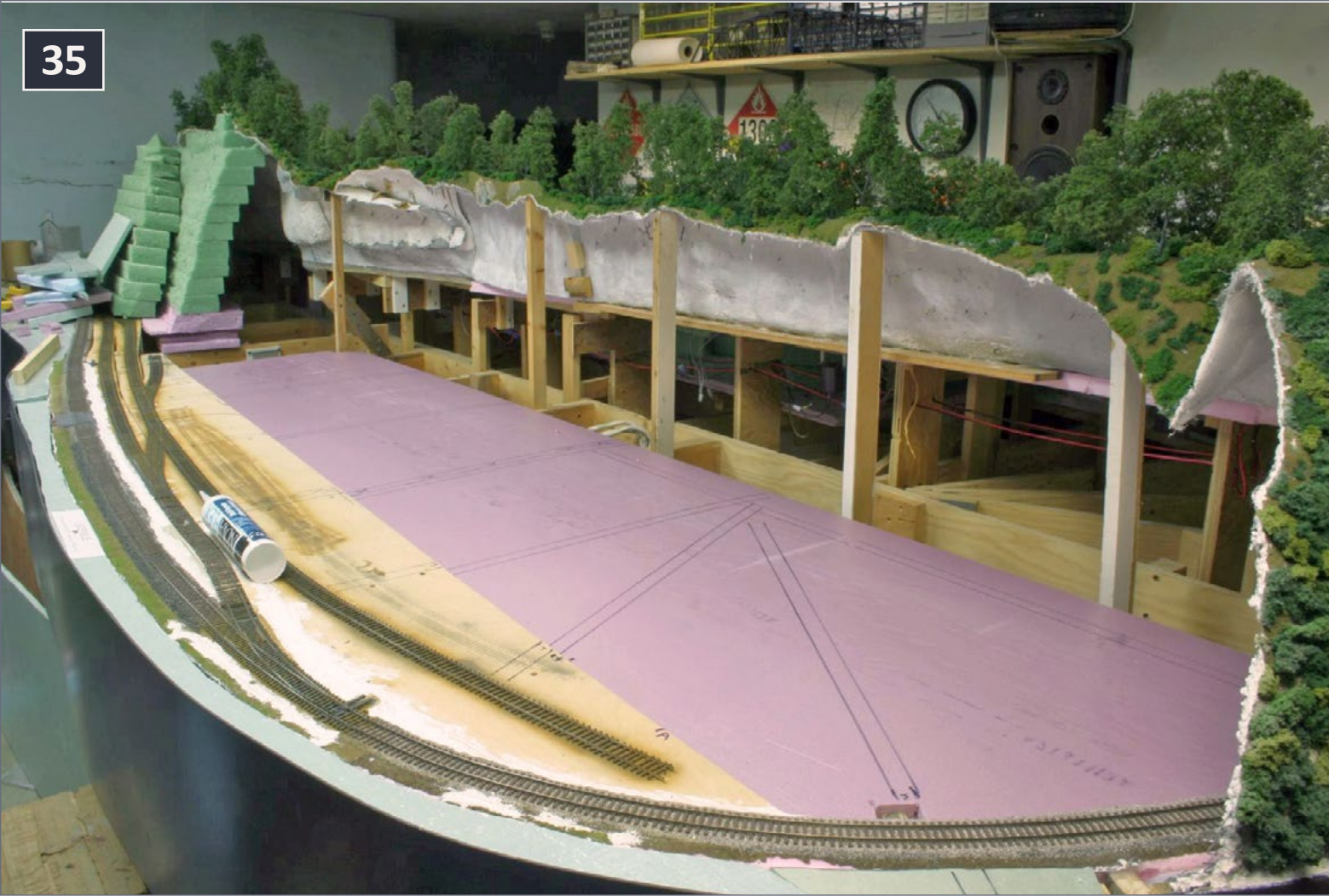
35. I removed the green foam overlay and carefully marked out the joist locations on the pink foam so that I could screw it down properly.
