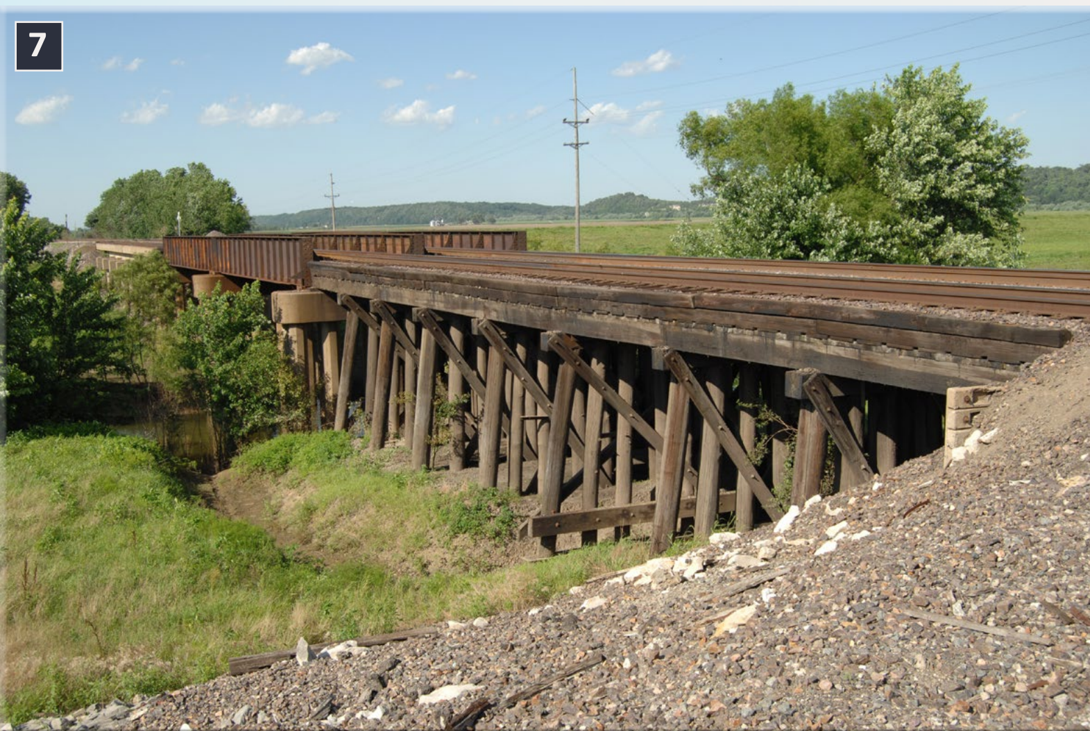
7. The wooden trestle supporting the approach span contrasts with modern segmental concrete work supporting the steel through-deck bridge. Dirk Reynolds photo.
