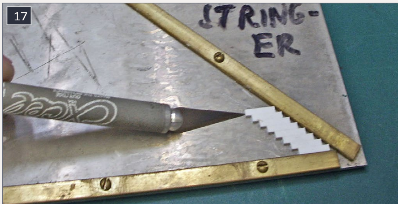
17. 4 x 8's are stacked against the edge of the jig until I have the desired height for the stairs.
