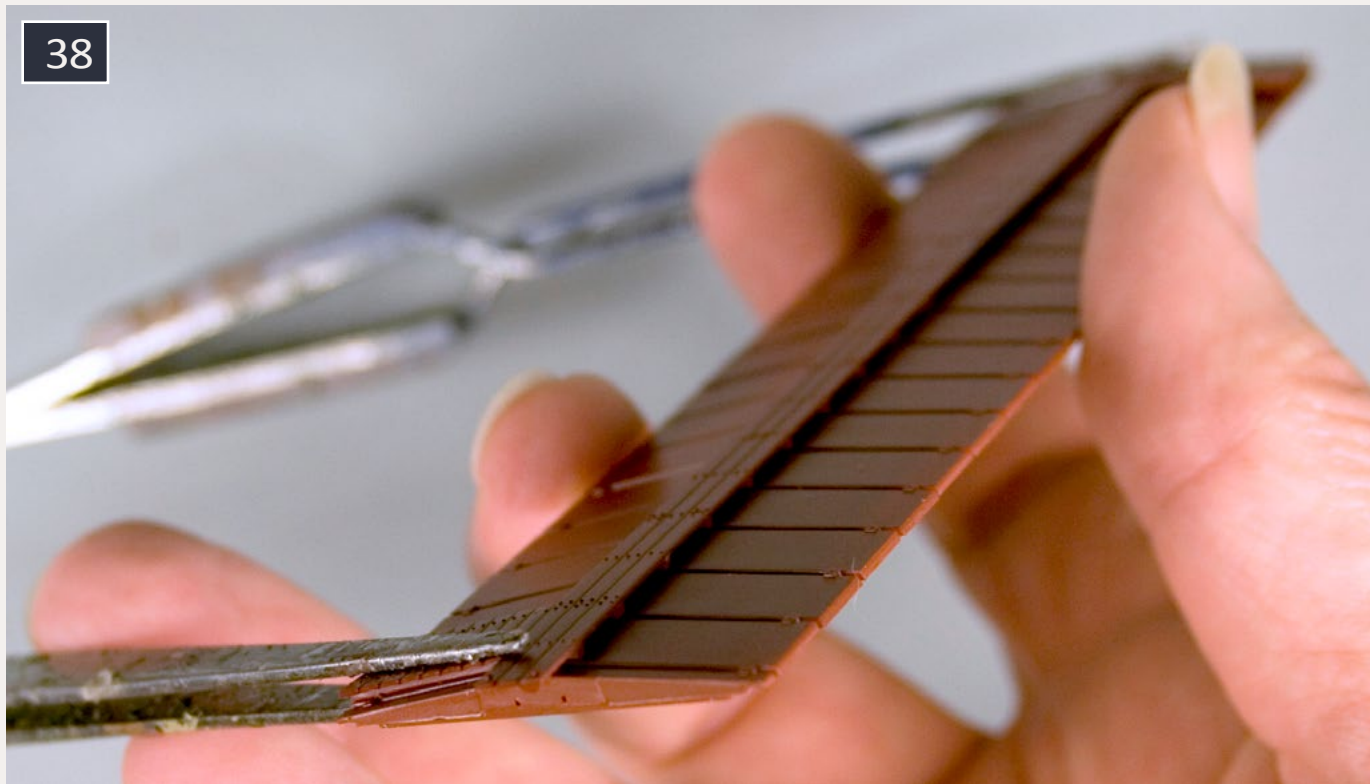
38: The running boards did not want to lie flat on a couple of the roofs, so clamps were necessary.
