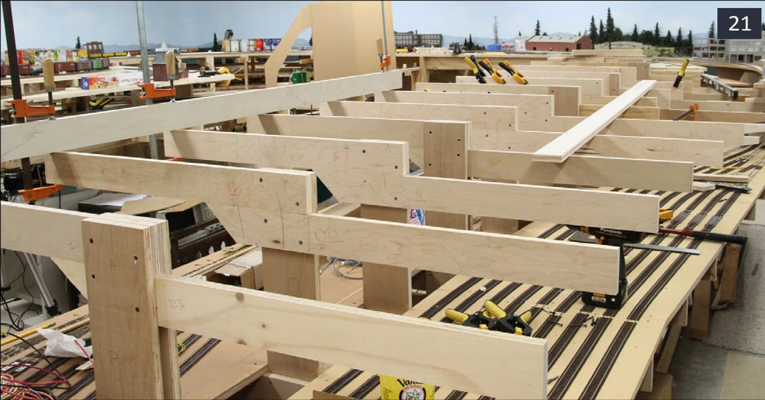
21: These risers and joists will support the peninsula's upper deck. The joists are assembled using woodworking biscuits. The backdrop will attach to the "back" of the joists and risers. "Photo circa December, 2013"
