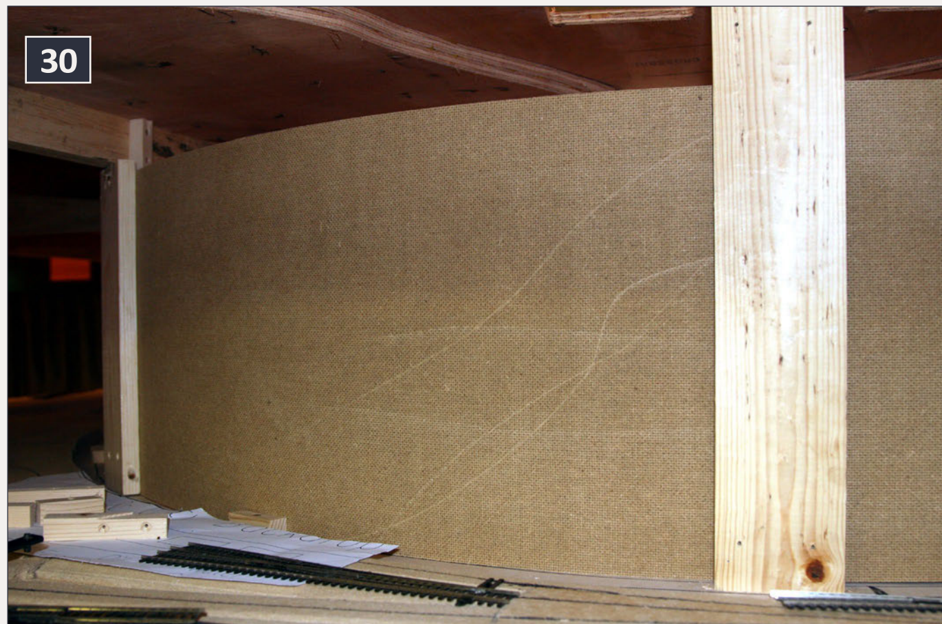
30: Backdrop supports between Shreveport and Watts.
